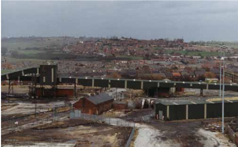
Gradual clearance of the colliery site From the Brierley Grimethorpe and Shafton Living Archive
